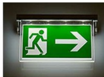
Signs & emergency light
