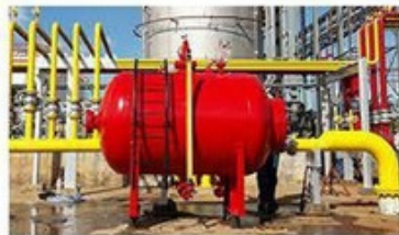
Foam Tank & Foam Equipment
